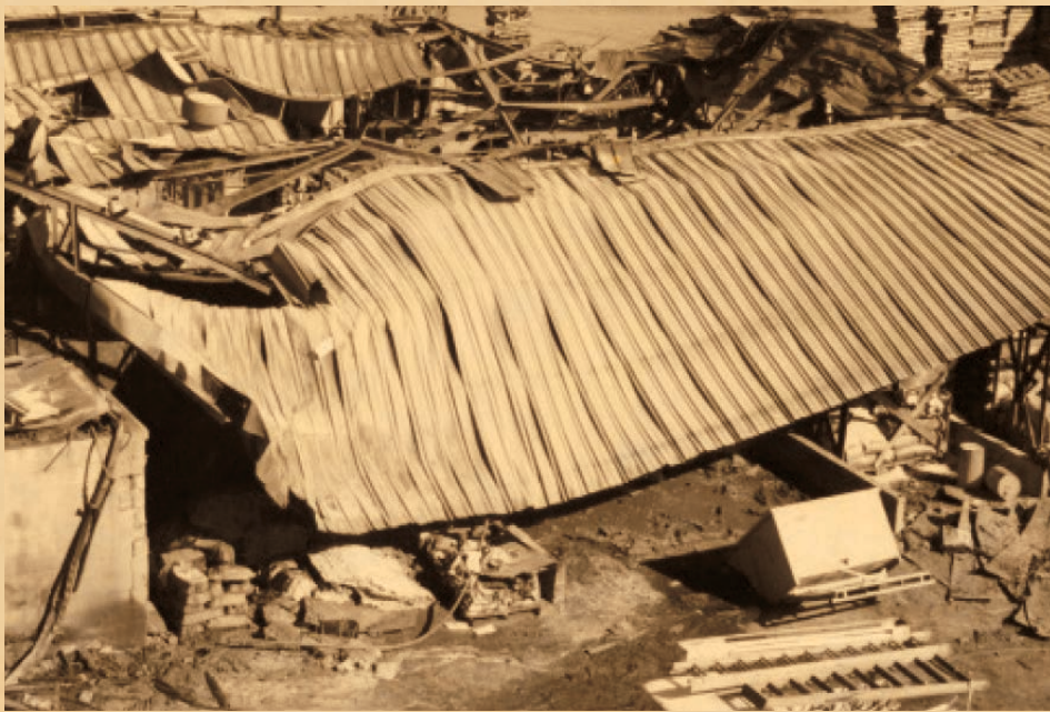
Roof collapsed over the mills due to Carson facility fire
